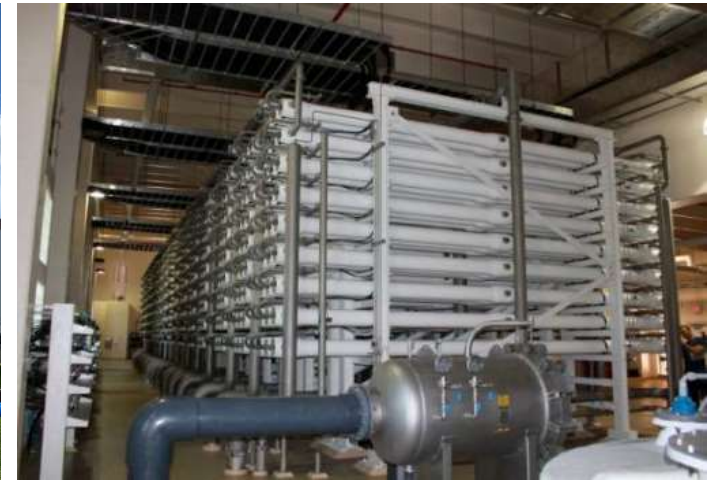
14.5 MGD Nanofiltration Process Constructed in 2010
