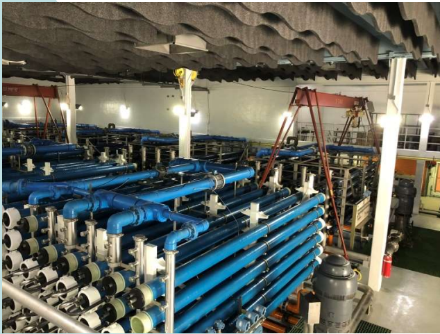
13.7 MGD Reverse Osmosis Process Constructed in 1990 Expanded in 1996 & 2005
