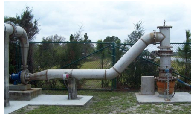
Floridan aquifer water supply well
