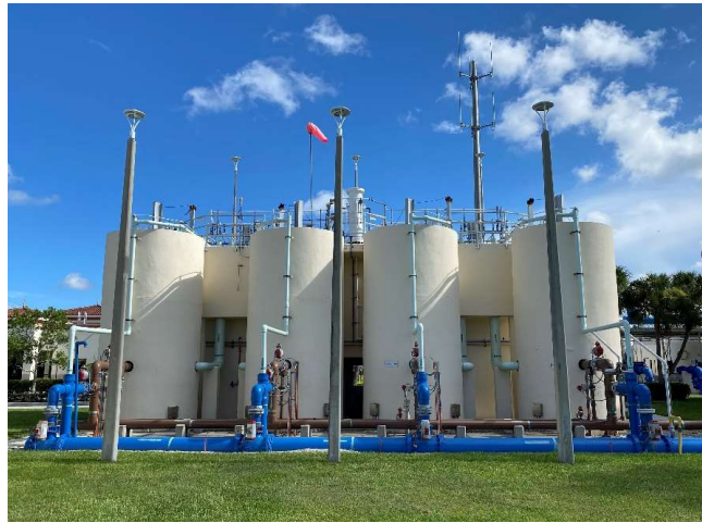
1.8 MGD Anion Exchange Process Constructed in 2000
