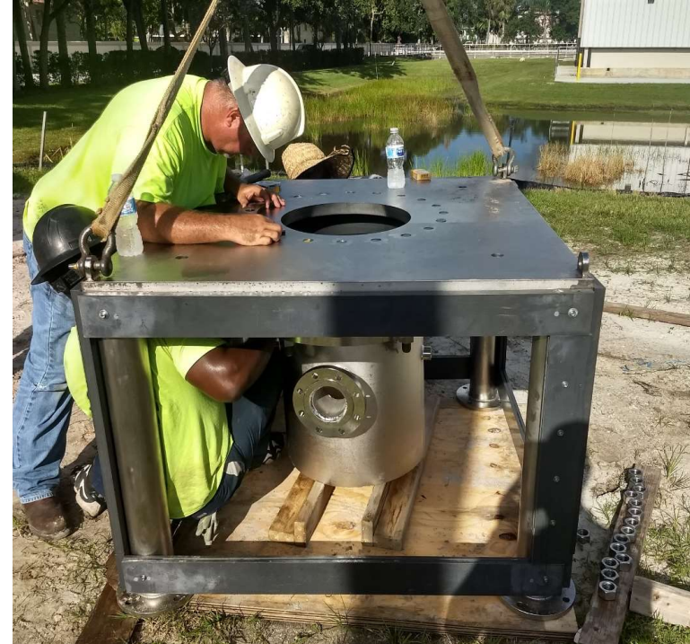
Wellhead support table and flushing tee
